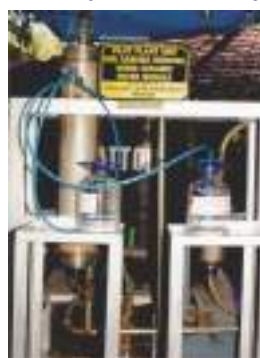
Pilot Plant for Arsenic Removal
